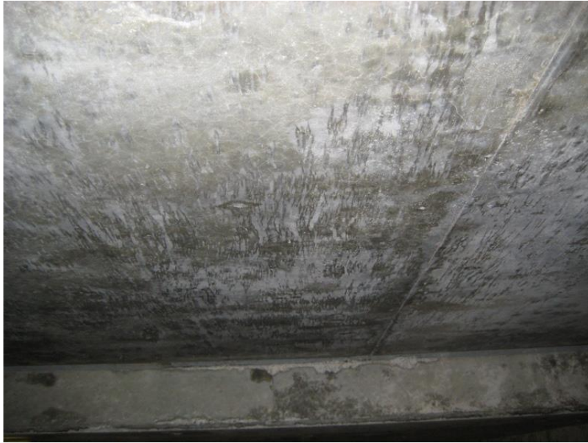
PLATE FOUR: Grain Imprint on concrete surface
