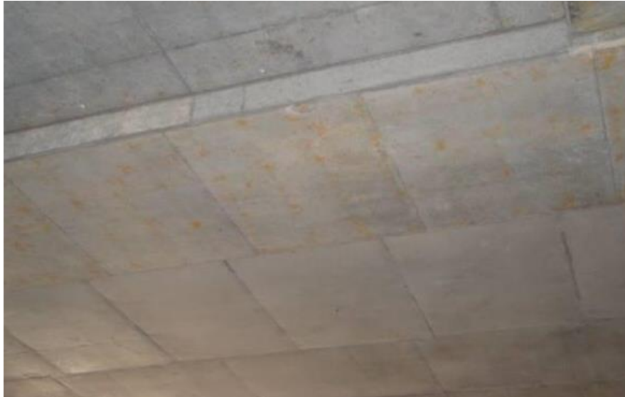
PLATE TWO: Rust Staining
